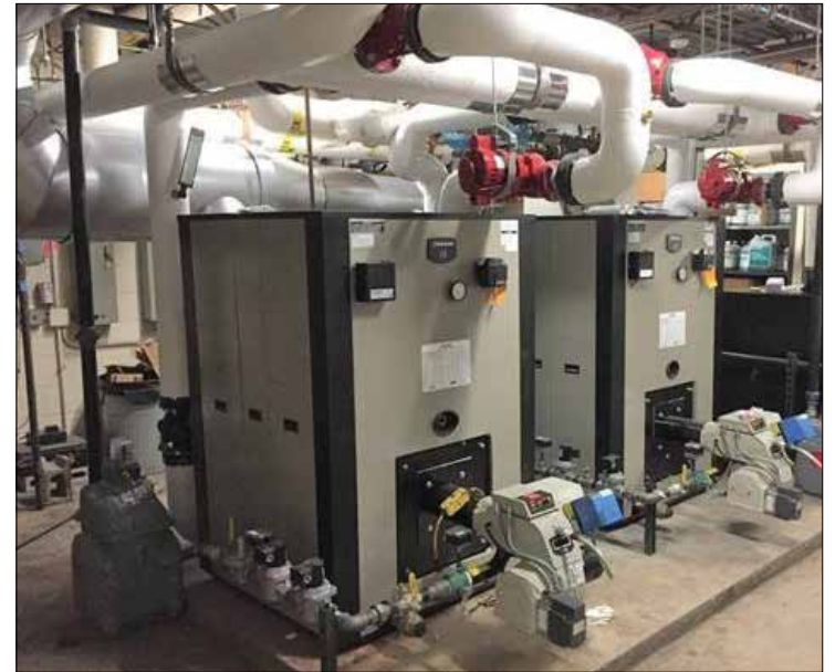
The boiler array ILNG project, one of the many commissioned by GTI Energy.
