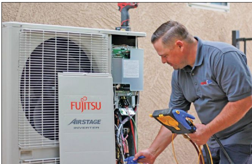
A SERVICE TECHNICIAN ATTENDING TO A FUJITSU AIRSTAGE VRF SYSTEM.
